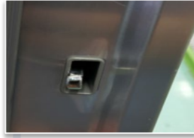
Misaligned door latch
