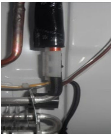
Sensor facing rear (incorrect)
