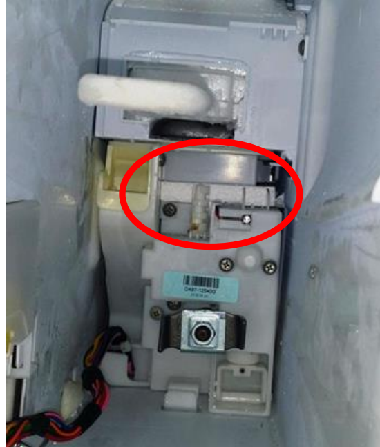
Auger Fan Blocked by Styrofoam
