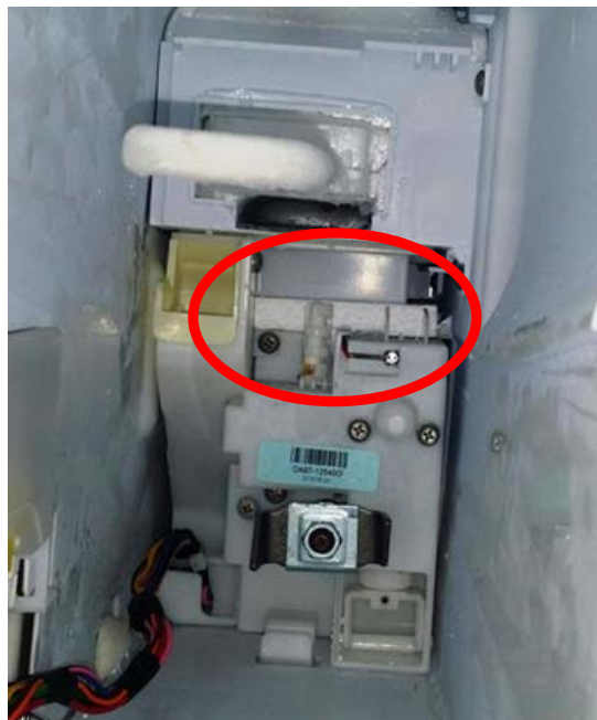
Auger Fan Blocked by Styrofoam
