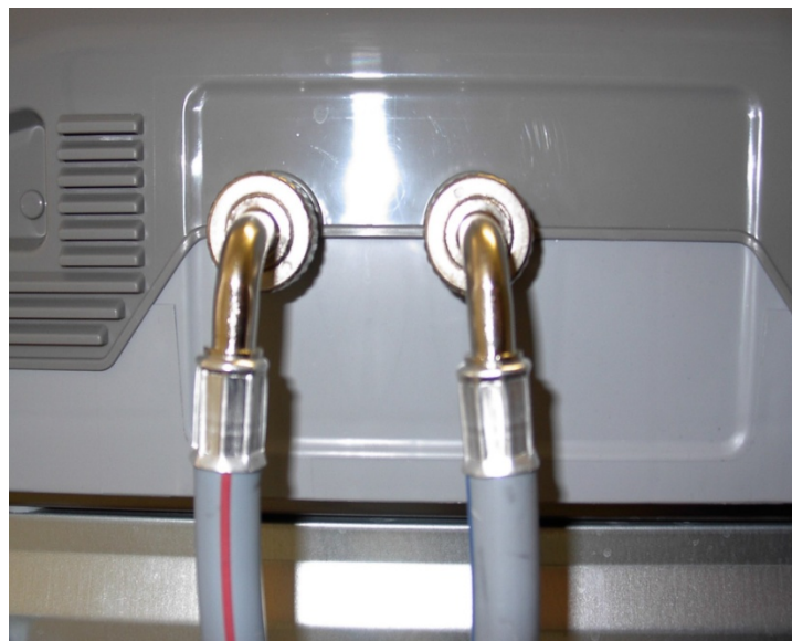
Water hoses at washer
